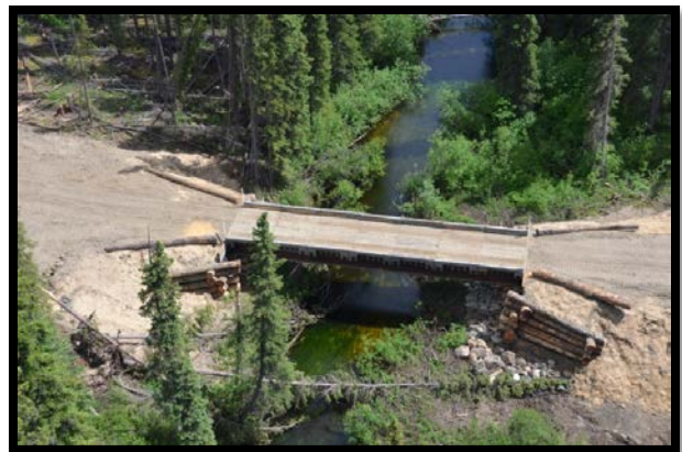
One of seven compliant bridges constructed by Carrier during the audit period.
